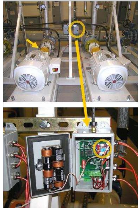
Figure 3: Sensors are mounted to analyze the vibration and assess the health of equipment at a semiconductor fabrication plant (picture is from [18])
